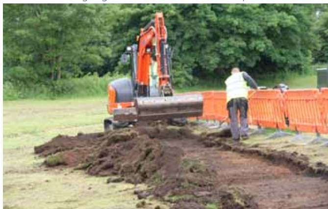
1. Well there's no going back now! The first level of top soil is removed.
