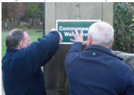
Installing one of the new signs at Comely Bank Cemetery in Edinburgh, which has 302 war graves. The signs can be erected on walls or railings or on a post near the cemetery.
