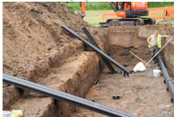
6. The serious business of getting it all in and level is under way.
