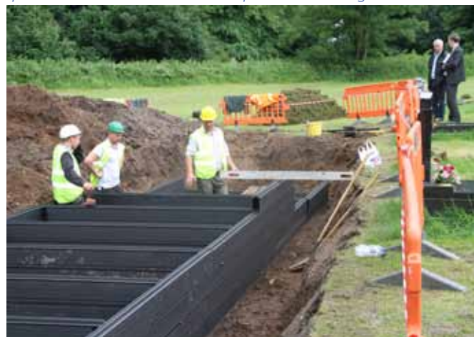
8. With the outer frame in and level the individual grave spaces are now being formed, 12 in total and the same dimensions as any other grave space 9' x 4'. As the units are built up so the backfilling continues.
