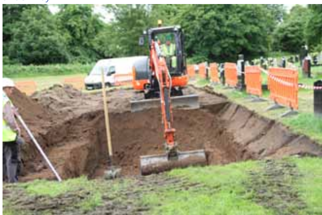
5. It's now late on Monday morning and serious excavations are well under way.
